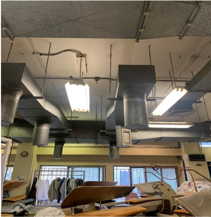
Overhead Ventilation System at the Laundry
